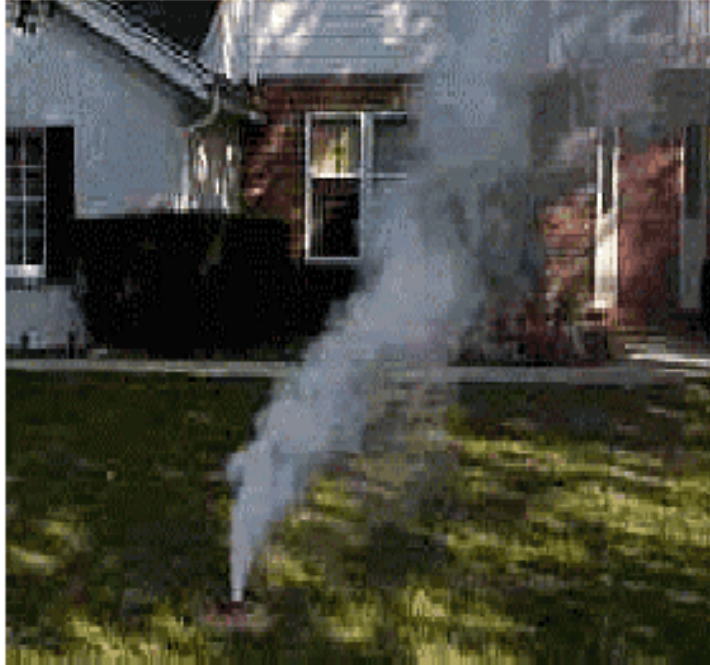
Figure 8-1 Smoke Escaping From an Uncapped Lateral Cleanout
